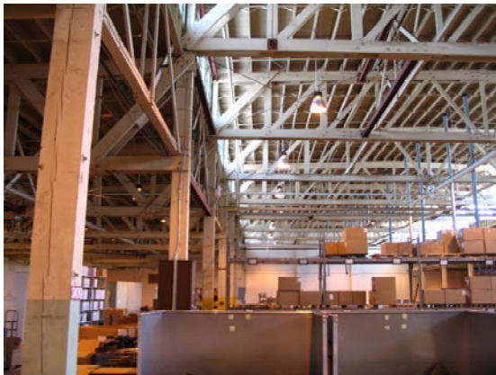
Ft. Lewis Timber Roof Truss Inspection, Ft. Lewis, Lacey, Washington; Cooper Zietz Engineers, Inc. for U.S. Army Corps of Engineers
